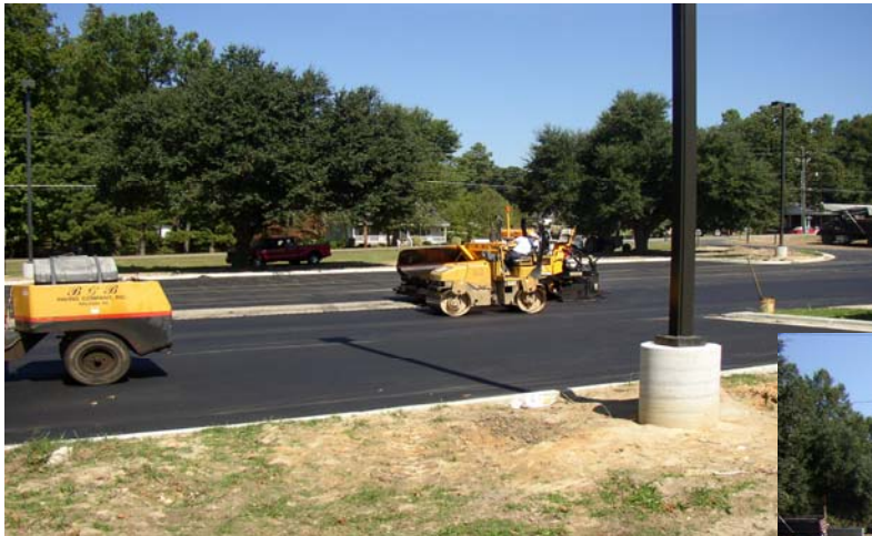
The Louisburg High School parking lot was nearing completion at lunchtime Tuesday (photo left and below).
